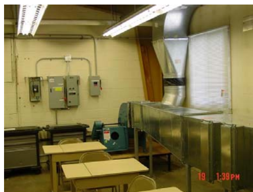
Newly remolded TAB Lab with digital, variable frequency fan controls
