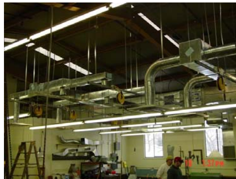
New TAB duct work and VAV control system.
